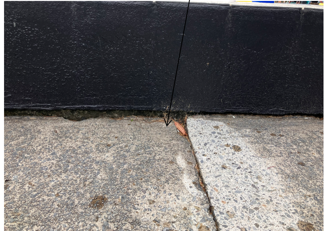
Slab on grade subsidized on the west side of the leisure pool. Top of concrete was ground flush to avoid tripping hazards.
