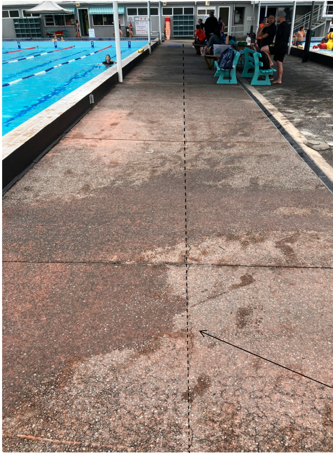
Slab on grade crack runs the length of the lap pool on the north side.
