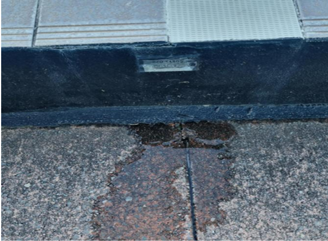
Fig 1. Half way down Lap (QE2 side) at scupper take of location water coming up through bulkhead/concourse
