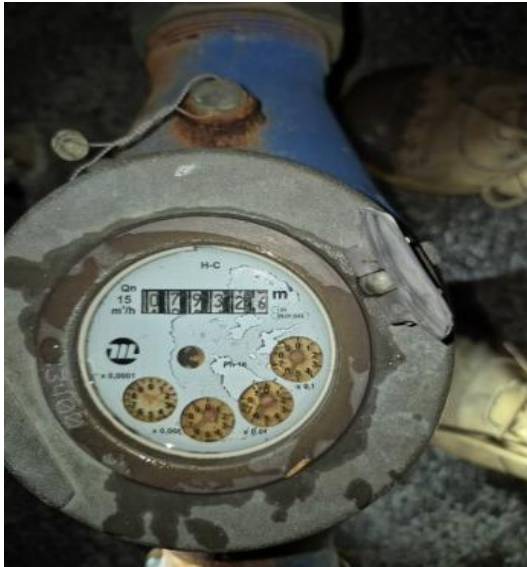
Water meter: 79393 (10.06.25) 18 hrs (67 m 3 mains water make up)
